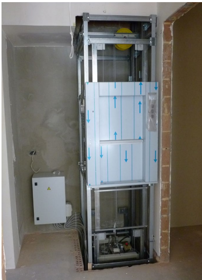
Top floor showing Control Box.
